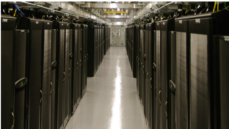
Massachusetts Green High Performance Computing Center (mghpcc.org)
